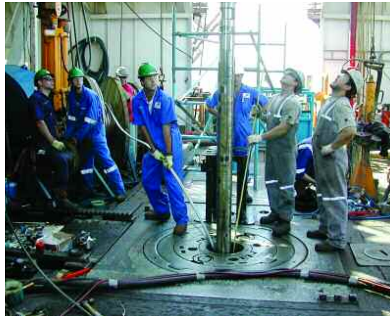
Centrilift dual-ESP systems are deployed in Santos' Mutineer and Exeter subsea tie-backs to an FPSO, offshore Western Australia
