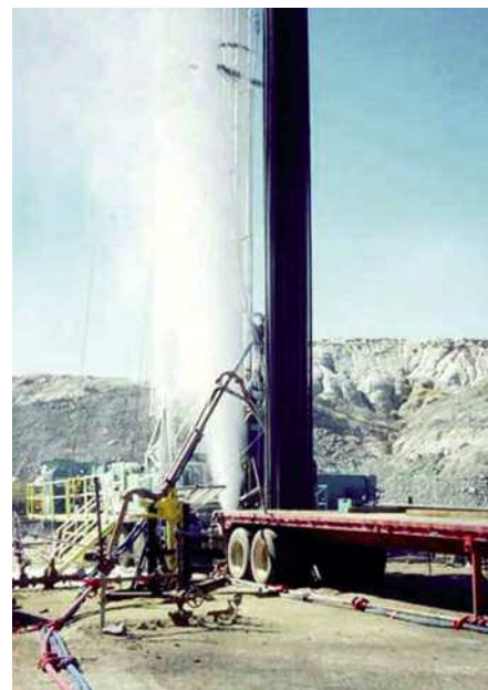
Taken at an actual site, this photograph shows how the FSR restrains a flow line, increasing safety on site. Notice how the high strength iron pipe was bent but was still contained by the FSR, preventing it from striking an active well to the side.
